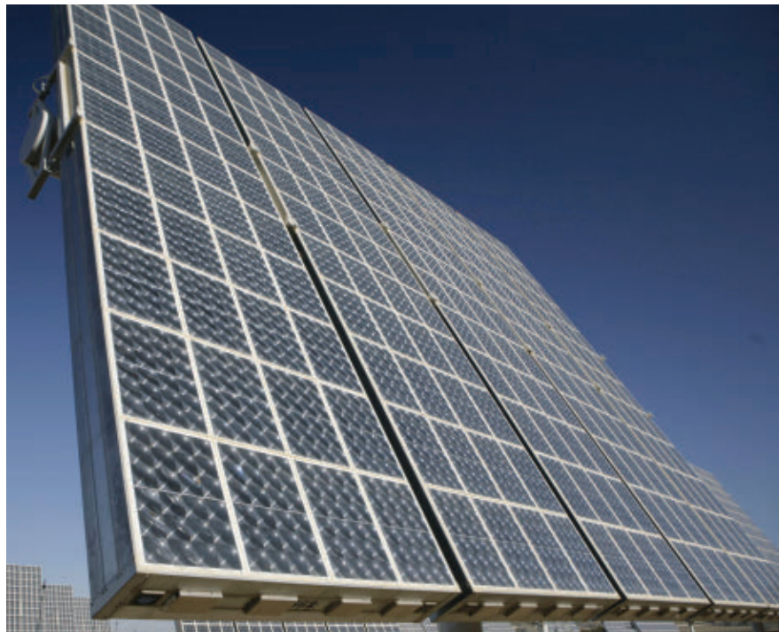
Concentrating PV is best suited for ground-based installations in the sunniest of locations, such as this site in Spain. Photo courtesy of Guascor Foton.
