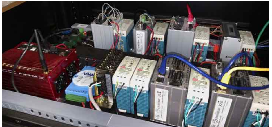
The WindCapture system allows SCADA Solutions to quickly scale back power generation during periods of low demand.
