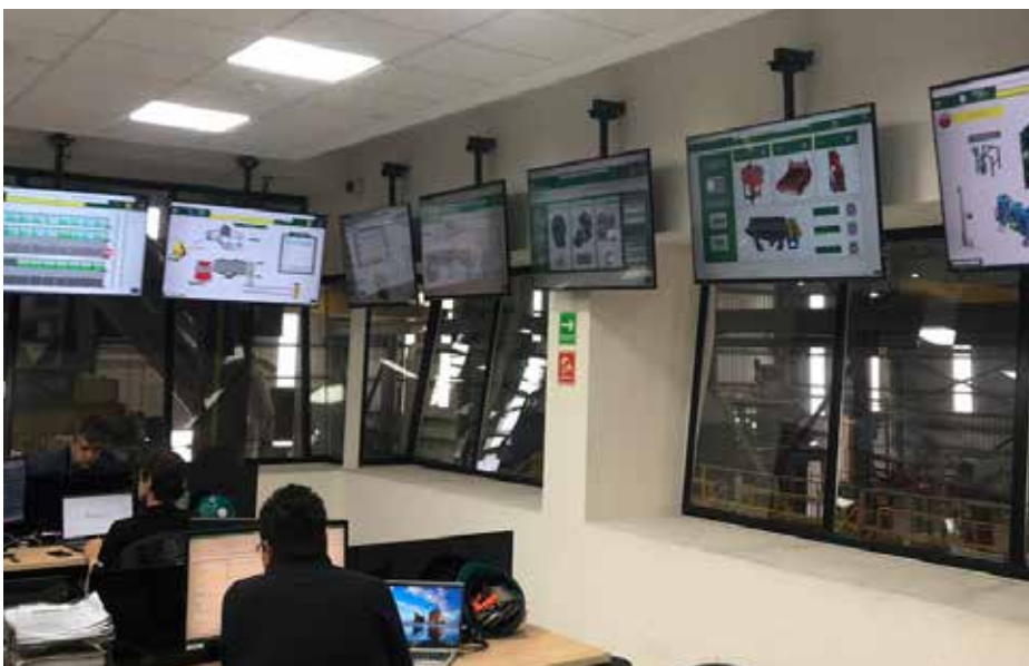
Ignition Perspective HMI screens in the main control room.
