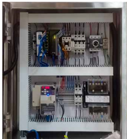
NACI manufactured VFD control panels for local conveyor control using Opto 22's groov RIO.
