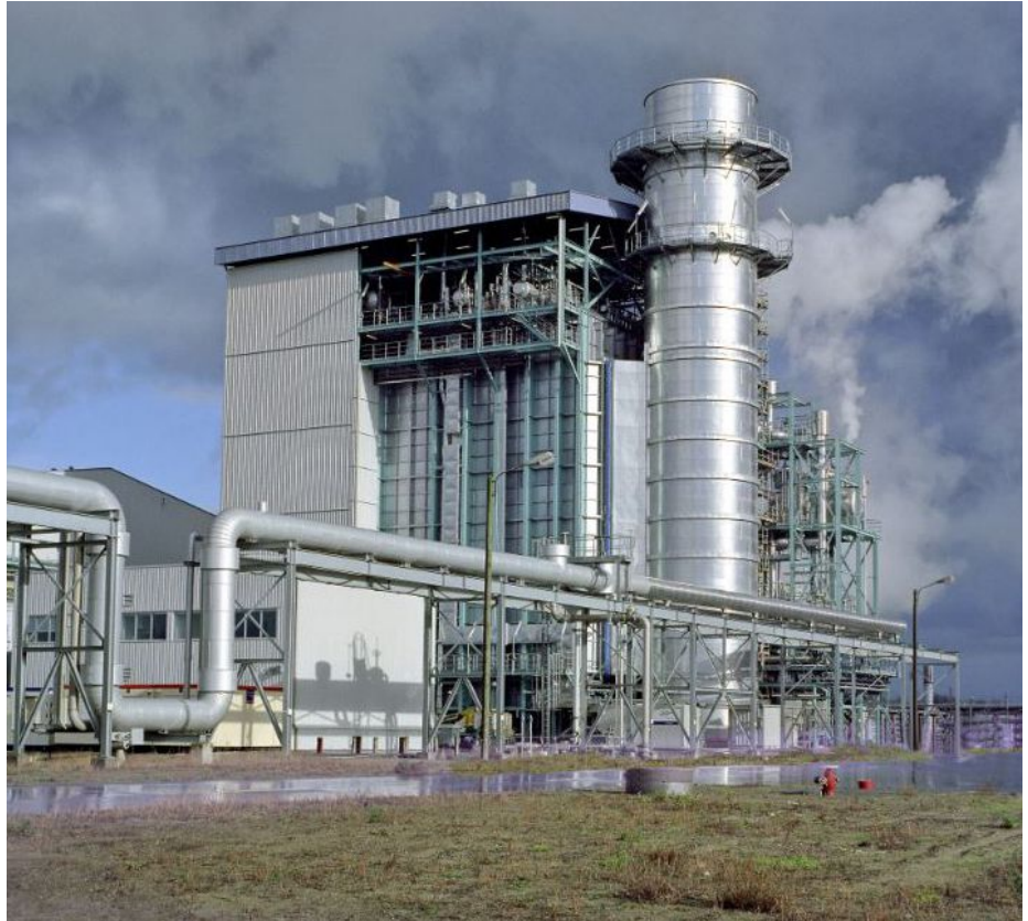
The automation solution integrates 16 plant clusters with different network infrastructures. One user group for each plant cluster enables access to devices and monitoring performance in private.
