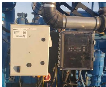
Pump and smart pump controller (side view)
